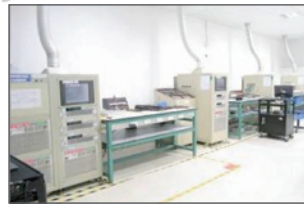
Electronic Load Testing Equipment (CHROMA) / 电子负载测试机组 (CHROMA)
